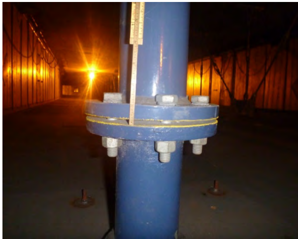
Figure 4.43 – Sign support with gaps at connection.
