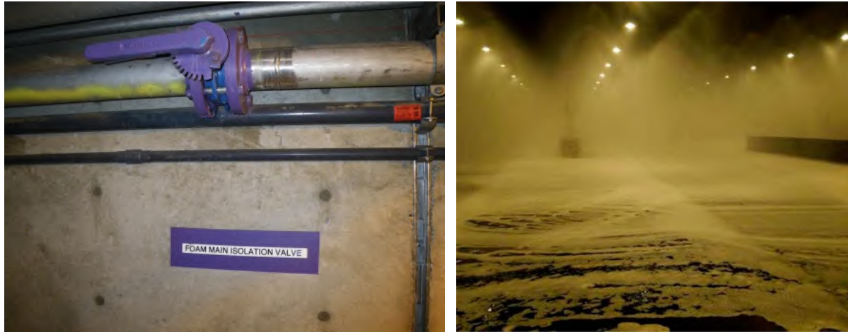
Figure 4.73 – Foam sprinkler system test.
