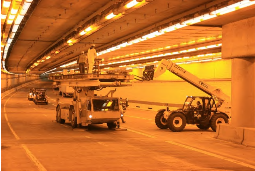
Figure 4.68 – Maintenance and inspection of lighting system.
