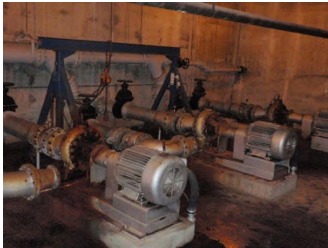
Figure 4.59 – View inside pump room.
