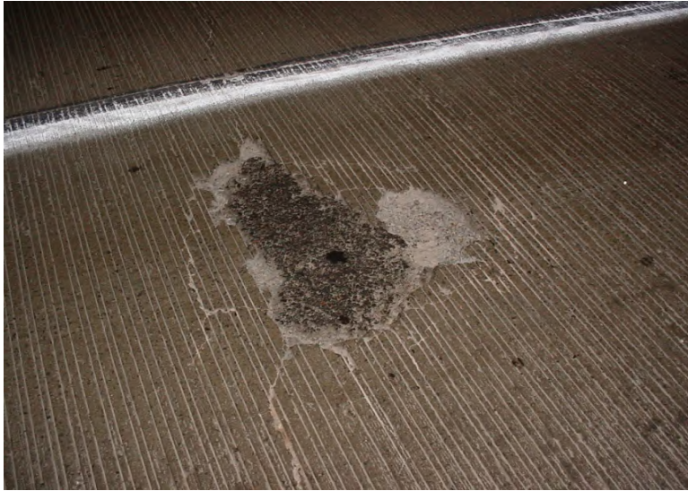
Figure 4.47 – Pothole with cracking in concrete wearing surface.
