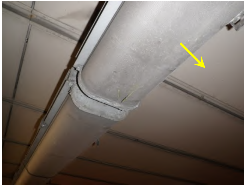
Figure 4.70 – Light fixture with damaged lens.
