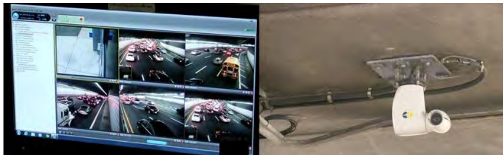
Figure 4.74 – Examples of CCTV camera systems.
