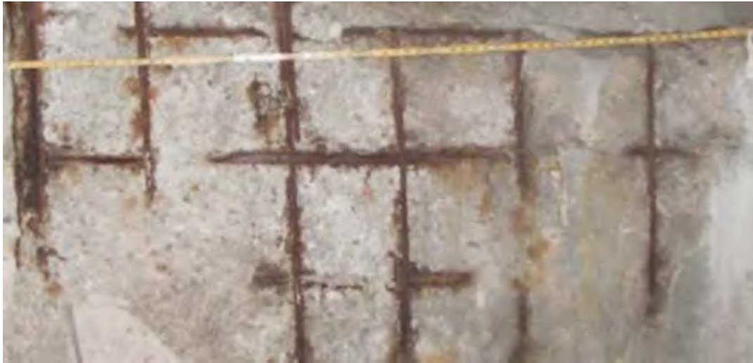
Figure 4.15 – Concrete spalling with exposed reinforcing steel.
