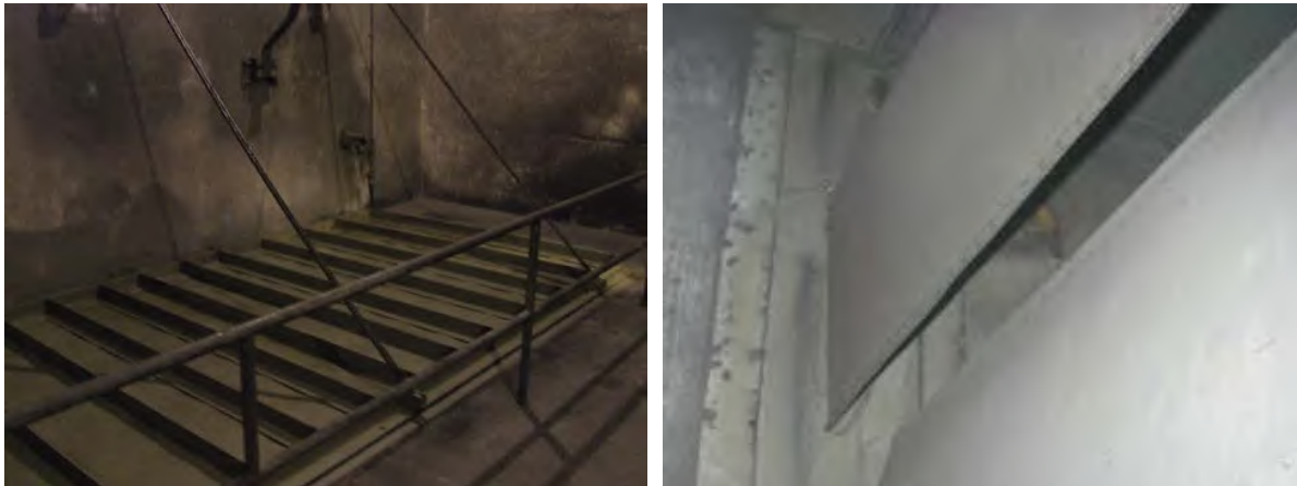
Figure 4.57 – Louvers in closed position, left; louver with large gap when closed, right.
