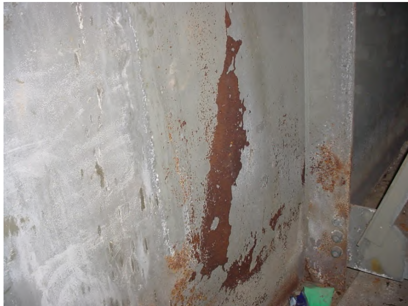
Figure 4.13 – Minor corrosion along roof girder.
