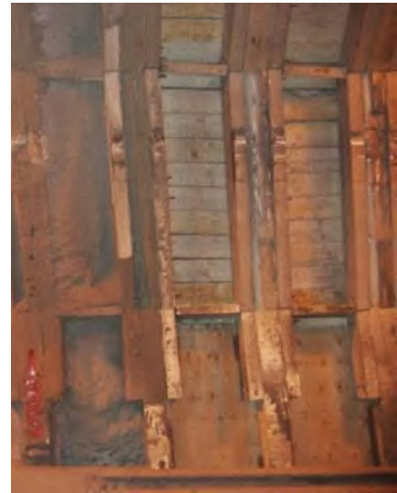
Figure 4.26 – Timber liner in state of deterioration.
