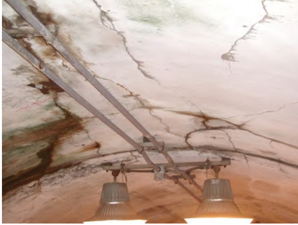
Figure 4.21 – Cracks with rust stains.
