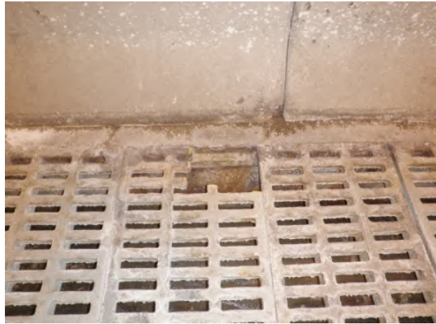
Figure 4.58 – Broken scupper grate.
