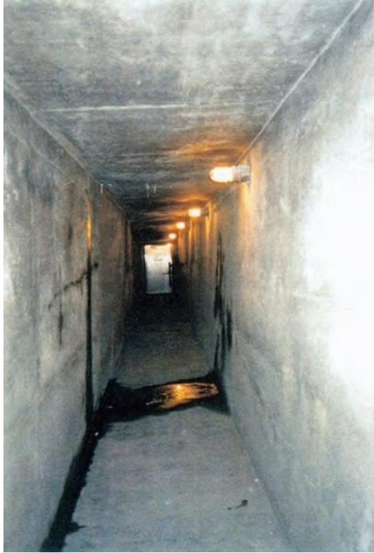
Figure 4.31 – Emergency corridor with minor leakage.
