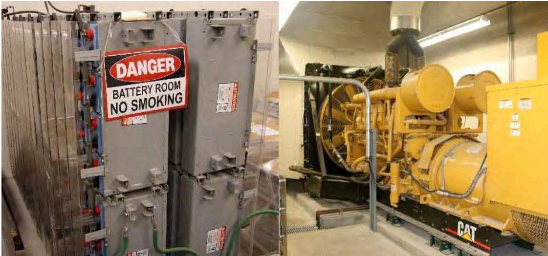
Figure 4.67 – Emergency power supply.
