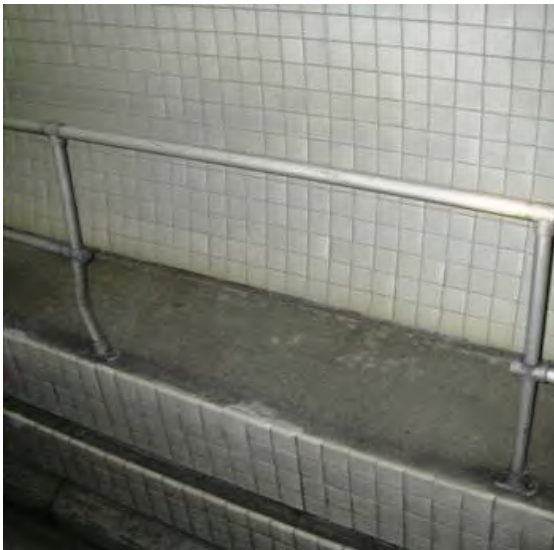
Figure 4.49 – Bent post and missing mid-rail.
