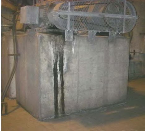
Figure 4.52 – Staining on the fan pedestal is evidence of lubrication leak.
