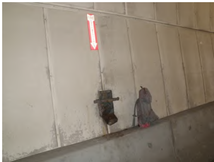
Figure 4.72 – Missing fire extinguisher.
