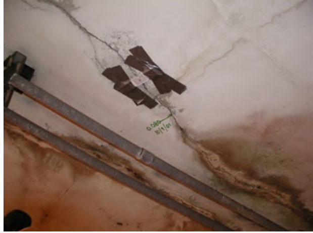
Figure 4.22 – Medium width crack in concrete liner.
