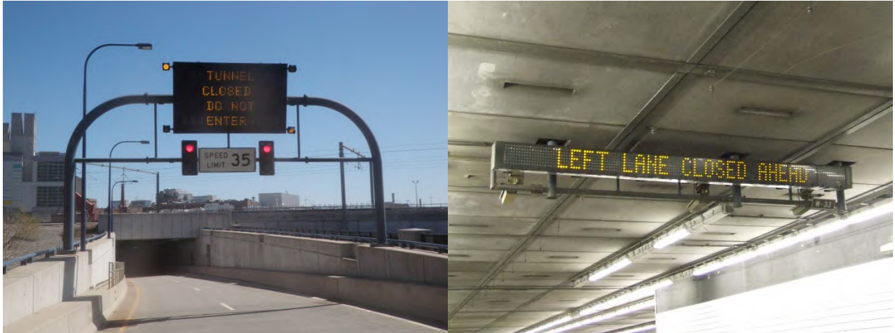
Figure 4.79 – Typical variable message boards.
