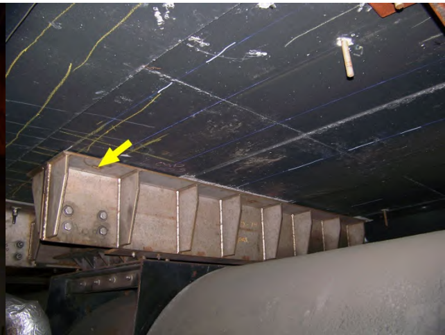
Figure 4.44 – Missing bolt at longitudinal fan support.
