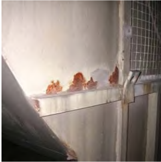
Figure 4.54 – Corroded fan housing.
