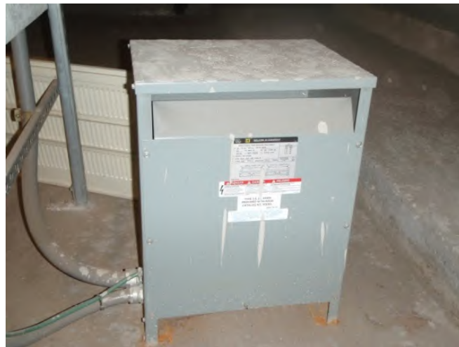
Figure 4.66 – Electrical equipment: Single phase insulated transformer.
