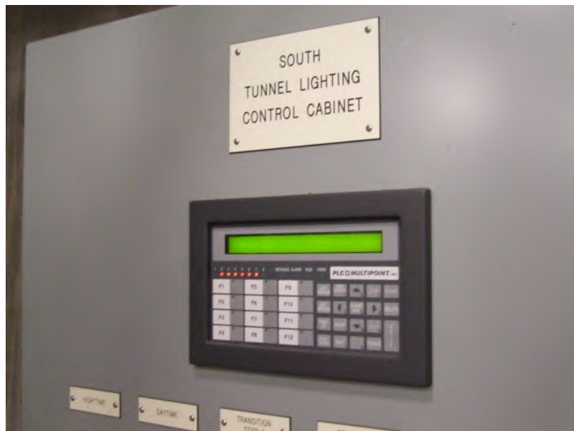
Figure 4.69 – Lighting control cabinet.
