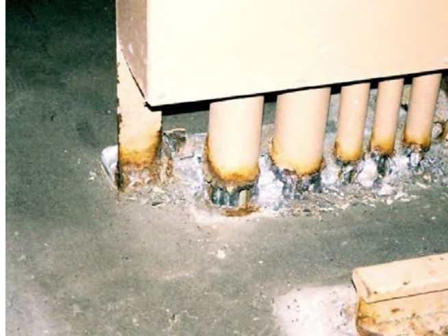
Figure 4.65 – Electrical conduits with heavy corrosion and section loss.
