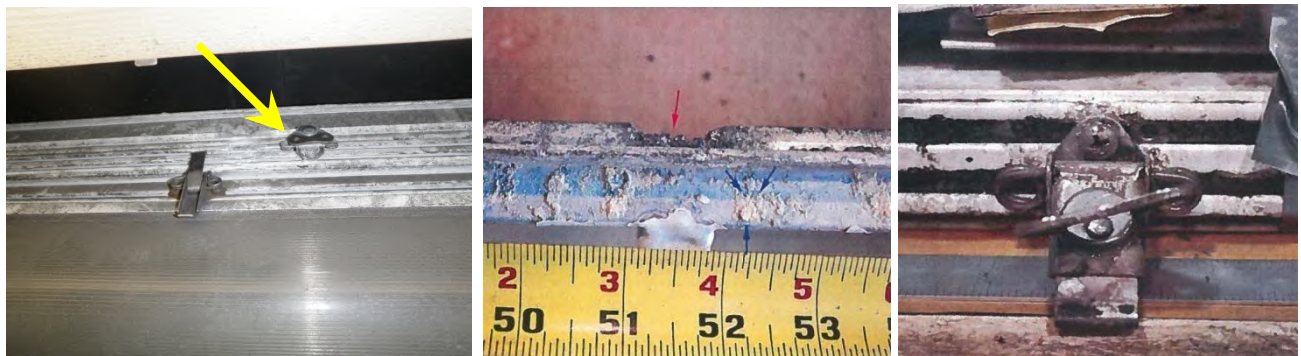
Figure 4.71 – Stainless steel clip severely corroded due to galvanic action.
