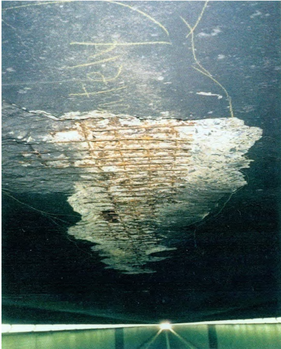
Figure 4.38 – Delaminated and spalled concrete with deteriorated and exposed reinforcing steel on underside of concrete ceiling slab.
