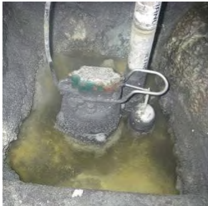
Figure 4.61 – Accumulation of calcium deposits at sump pump.
