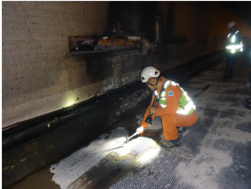
Figure 4.6 – Evaluating fire damage.
