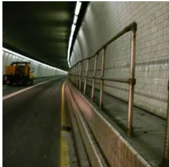
Figure 4.50 – Bent pedestrian railing with missing railing components.
